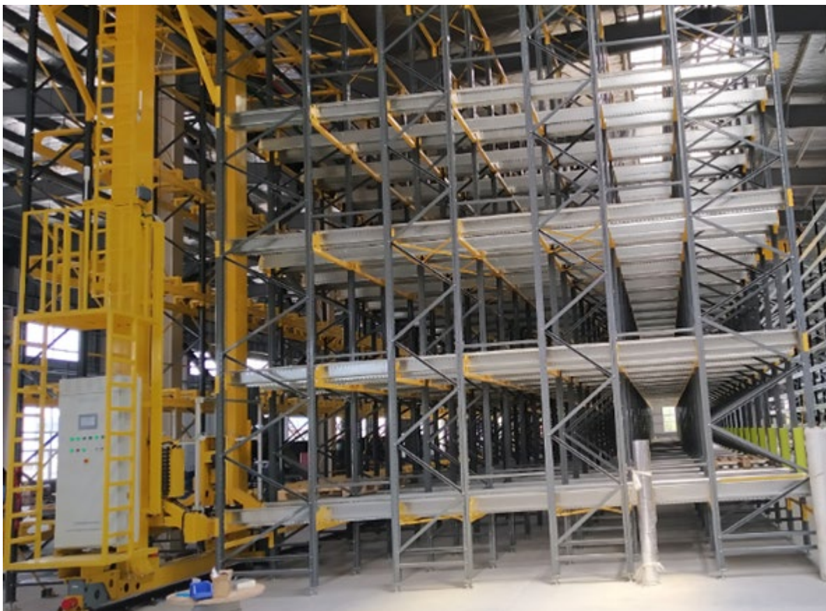
Stacker Crane + Pallet Runner System
